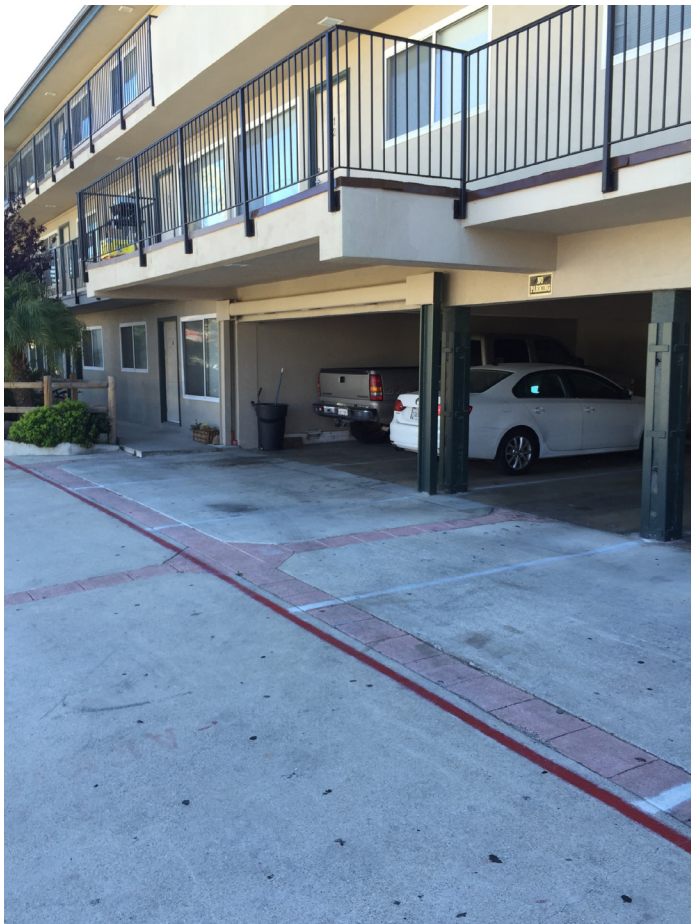
The Abrego Apartment has multiple stories above ground-level parking, supported by narrow vertical supports, making this an ideal location for installing Hardy Frame's SMFs.
